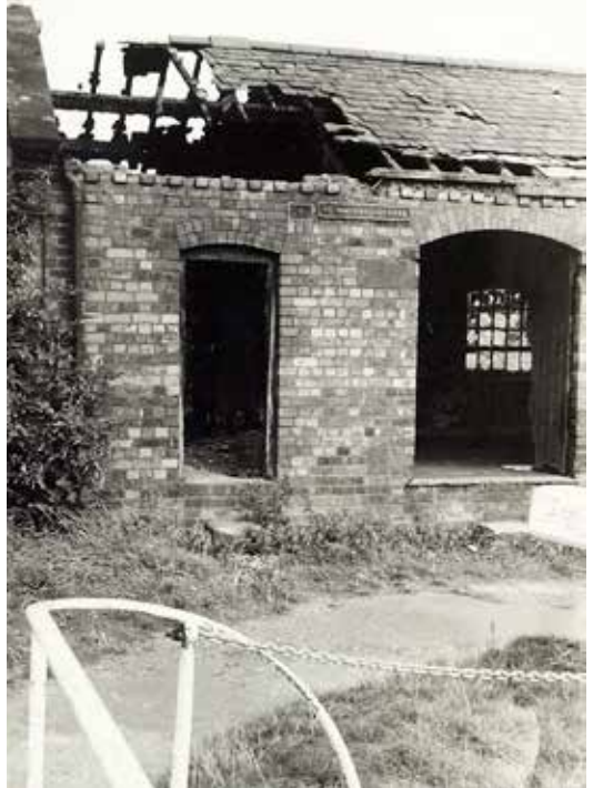
The fire-damaged Pattern Shop before restoration
